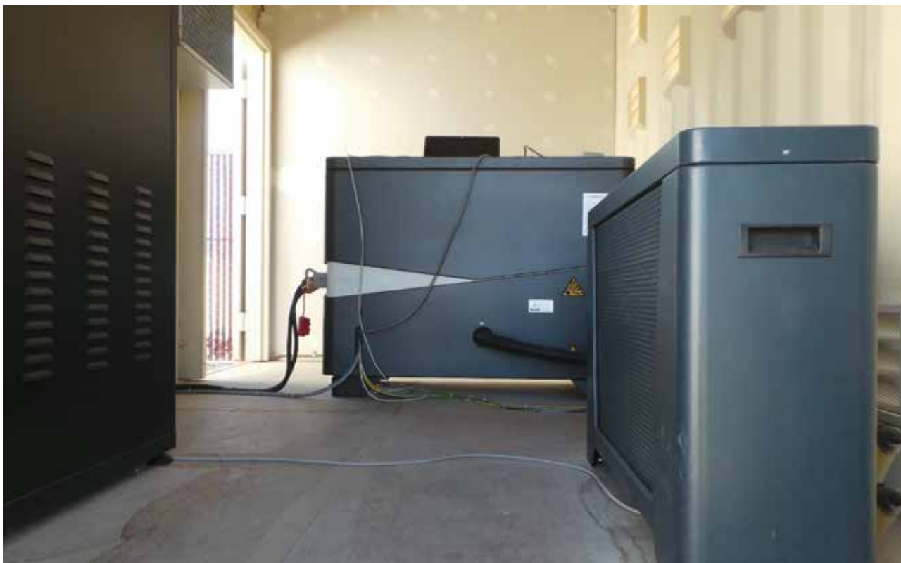
GenCell's G5rx back-up fuel cells installed at a substation for San Diego Gas & Electric (SDG&E). The fuel cell will automatically operate in the event the power grid goes down. The fuel cell can operate 10 times longer than existing back-up power sources, and has the capacity to maintain all substation operations versus only critical operations.
