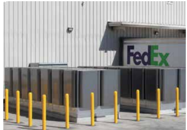
Bloom Energy's Bloom Server provides reduced emission resilient power from natural gas
