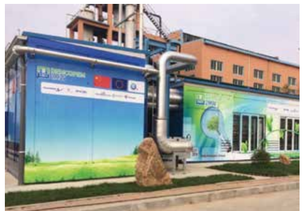
Nedstack has installed a 3.6 MW rated unit capable of delivering 2MW nominal electrical output and up to ~2MW in heat. The unit utilises waste hydrogen from the adjacent chemical process to produce heat and power.
